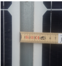
Al mounting rails between panels (spacing ~2.7cm)
